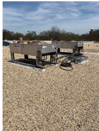
Figure 8: Existing Condenser on Roof
