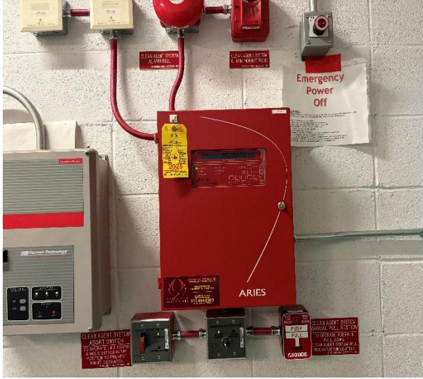
Figure 5: Dry Agent Fire Protection Control Panel
