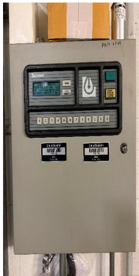
Figure 3: Existing CRAC Control Panel
