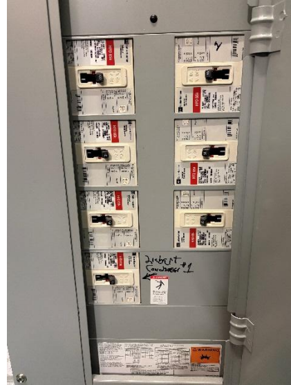
Figure 6: Existing 480V Distribution Panel
