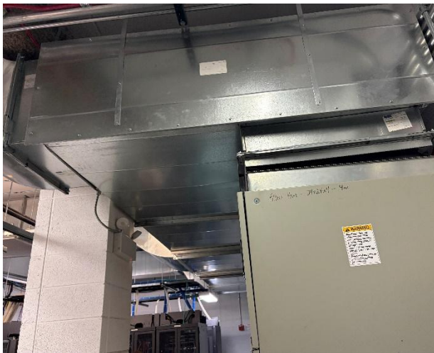
Figure 7: Overhead Return Duct Connection
